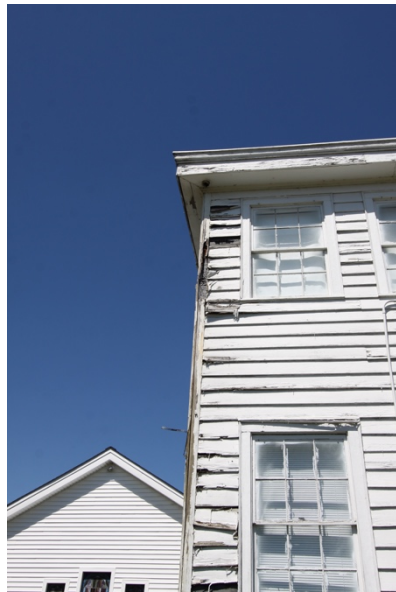
Figure 17 Paint loss and weatherization due to the disconnection of a downspout.
