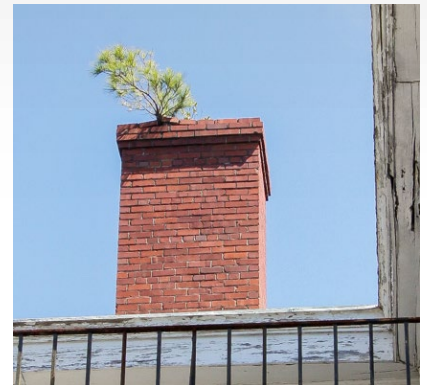
Figure 26 Vegetation that is protruding from a historic chimney.
