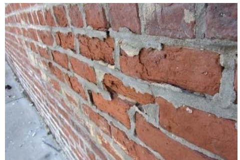
Figure 14 Historic masonry that has been repointed with Portland cement which has led to degradation.
